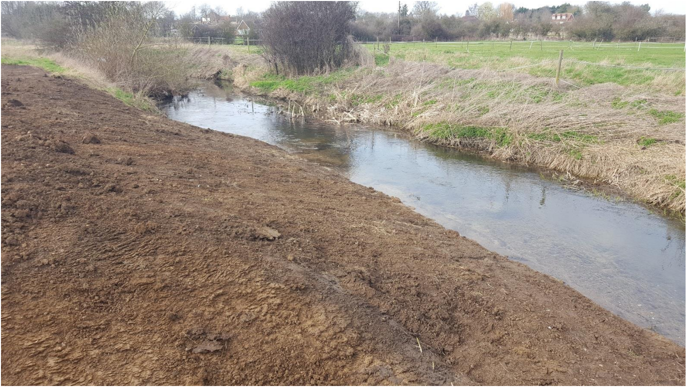
Photograph 2: Newly constructed berm to increase flow and habitat diversity on the River Chelmer at Springfield Nature Reserve.
